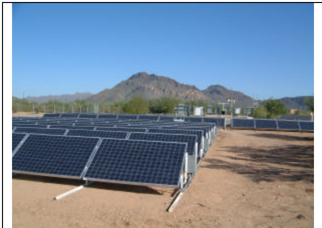
Another view of the two systems located at the Hayden/Udall water treatment facility.
