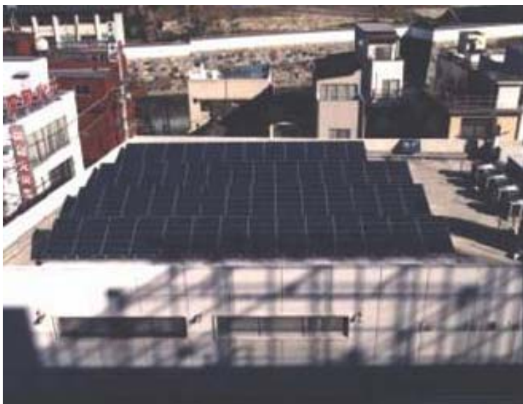
The commitment to solar by Tokyo Electric Power Company, the world's largest independently owned utility, is evident by the installations on several of its facilities, including its Yamanashi Branch office, above.
