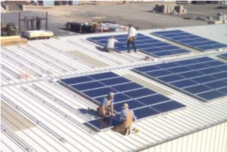
RWE Schott Applied Power completes the installation of the 30-kW solar electric system on Palmdale Water District's shop building.
