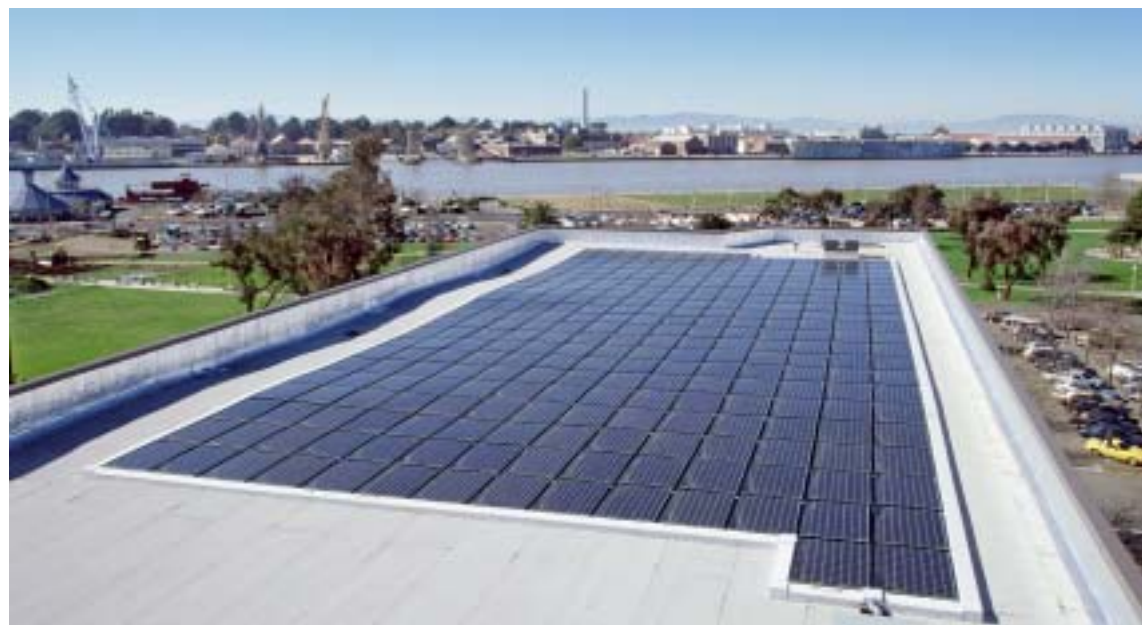
In March, the City of Vallejo, Calif., dedicated this solar electric system, located on the roof of the City Hall.
