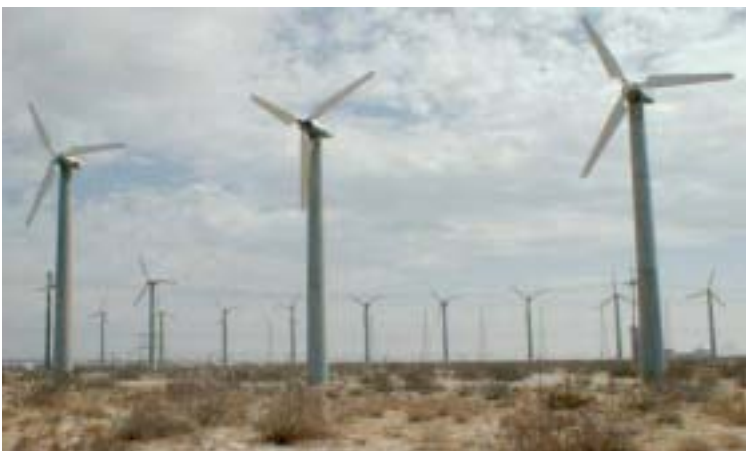
The South Coast Air Quality Management District, based in Los Angeles, California, in partnership with the U.S. Department of Energy, uses a hybrid wind-hydrogen system, powered by these three turbines.
