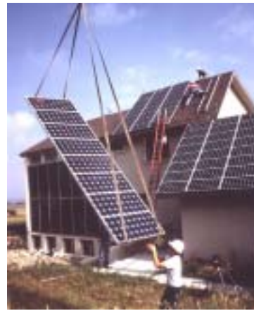
National standards for voluntary certification will help to ensure the safety and performance of solar electric systems.
