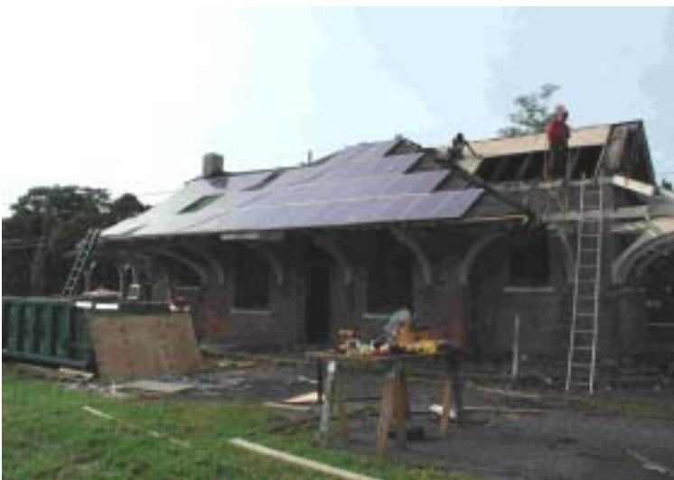
The Brentwood, N.Y., Railroad Station is being remodeled to accommodate the Fiesta Solar Café. A Kyocera solar electric power system was added to the roof and another to a parking structure.
