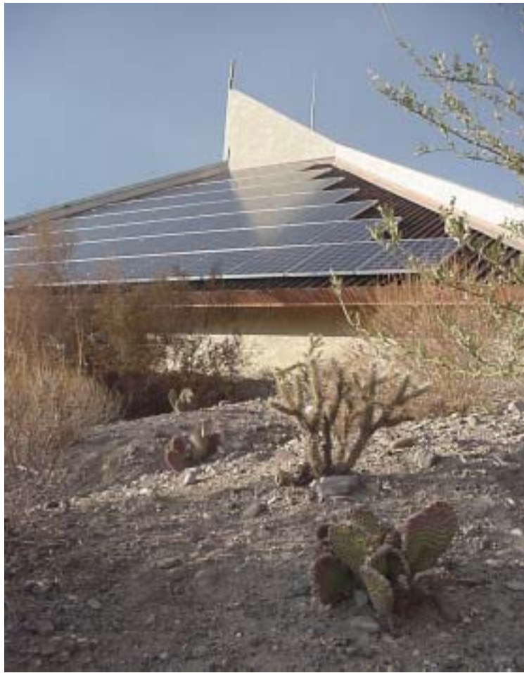
The Imperial National Wildlife Refuge features a 10-kW solar electric installation, designed and installed by American Solar Electric, with modules from Kyocera.
