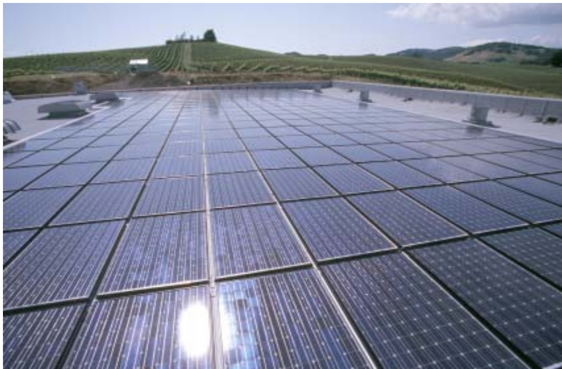
Challenging the Status Quo: The Domaine Carneros Winery in Napa Valley, California, features a 200-kW PowerLight solar electric system that supplies up to 40 percent of the winery's electricity needs.
