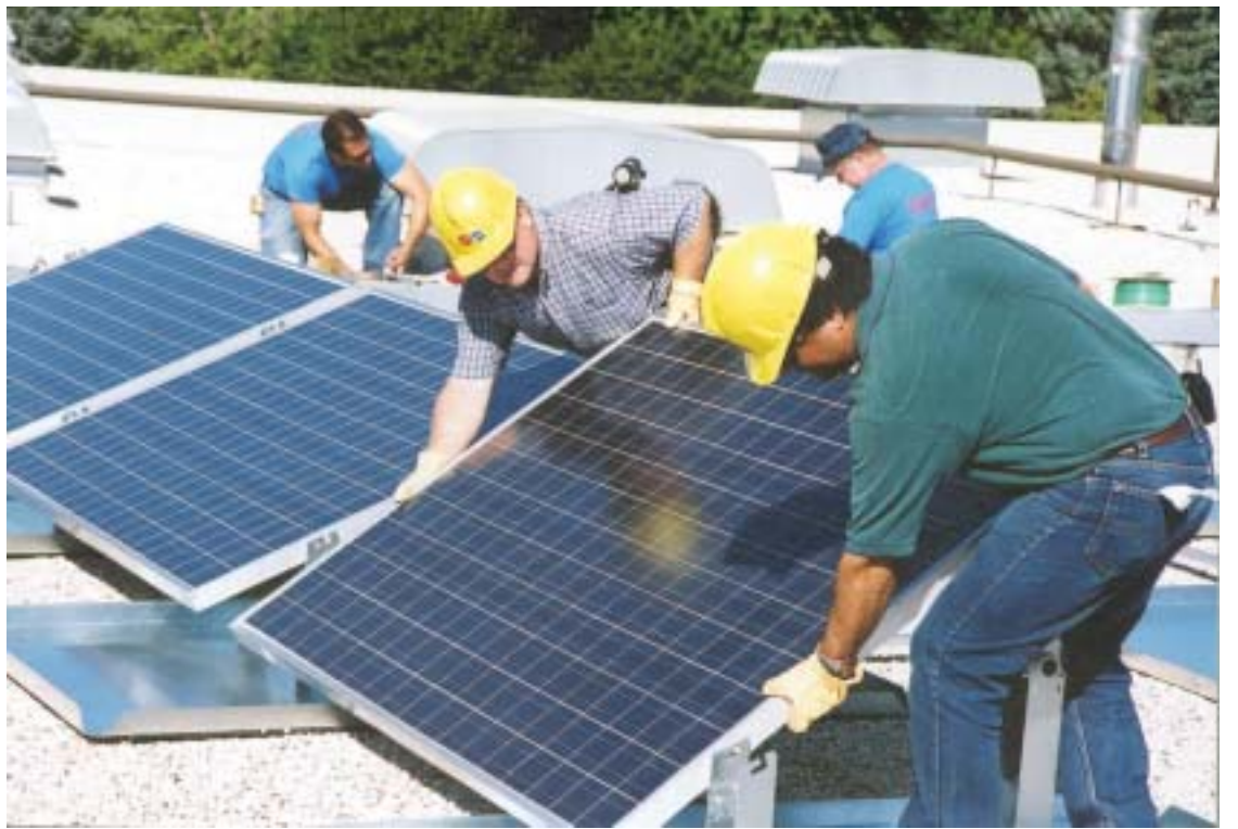
Local installers complete the roof-top solar electric system on Ashwaub High School as part of Wisconsin Public Service Company's SolarWise for Schools program.
